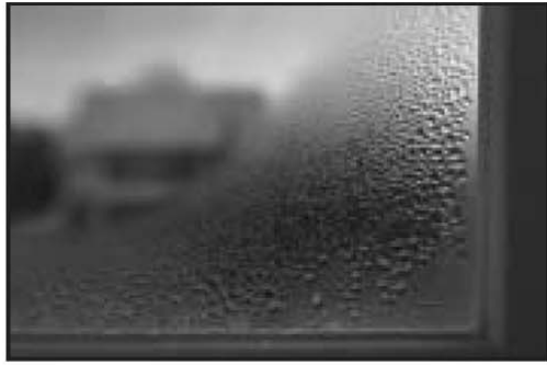
Condensation on the inside of a windowpane.
